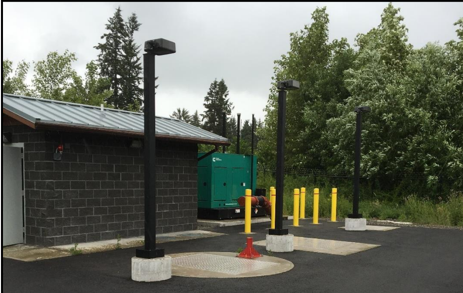
Lift Station No. 23
